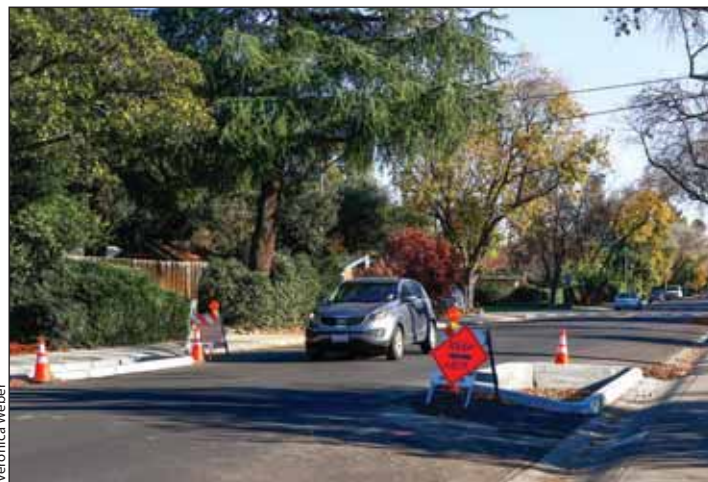
Concrete fixtures newly installed on Ross Road in south Palo Alto push both cars and bicycles into the same lane. The design is intended to slow traffic and make it safer for cyclists.
