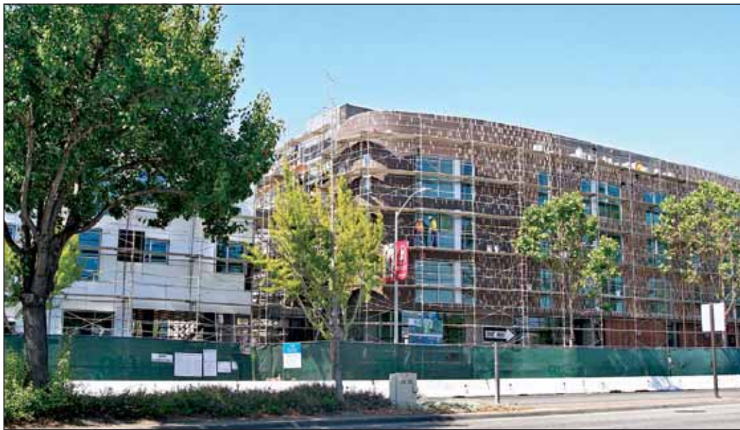
Construction workers add tiles to the exterior facade of Mayfield Place at 2500 El Camino Real, a mixed-use building that will have 70 below-market-rate housing units and is expected to be completed in October 2016.
