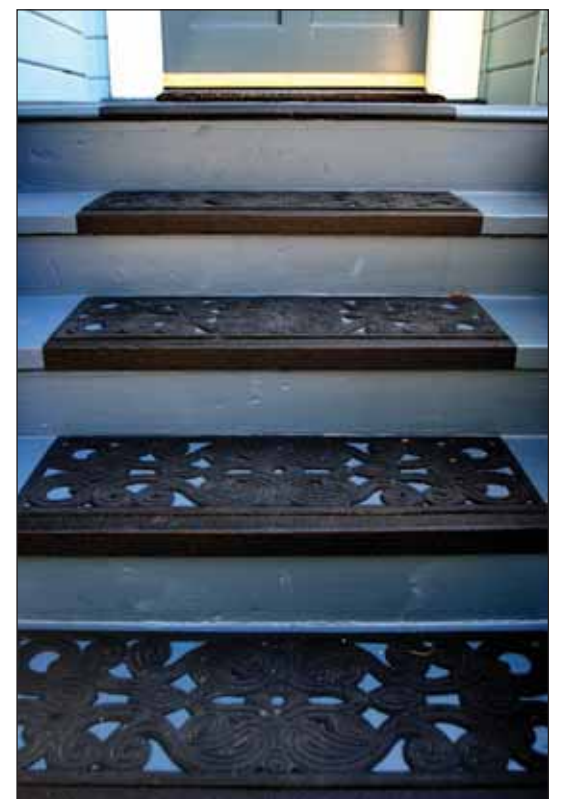
Skids on slippery steps can be prevented by installing decorative rubber mats (nailed down), as well as sandpaper, nonskid strips.
