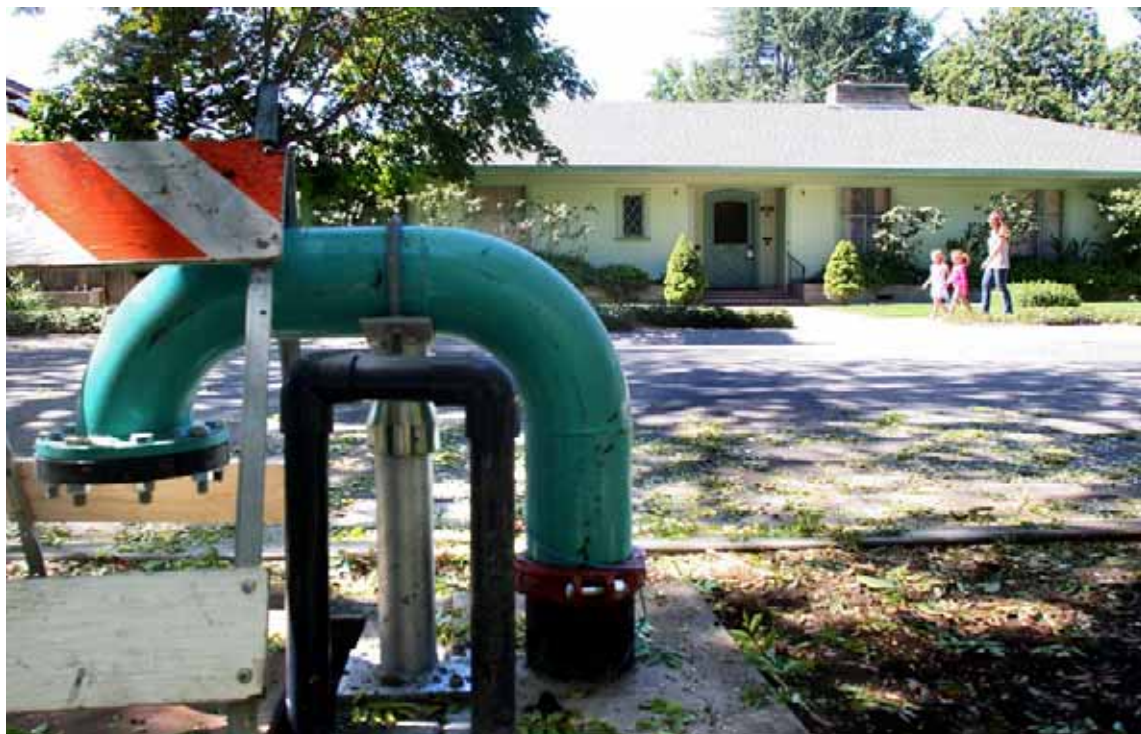
An underground well is being constructed at Eleanor Pardee Park to provide emergency-water storage.
